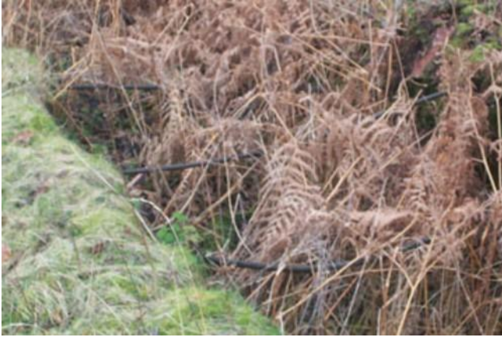
A surface depression, looking east
