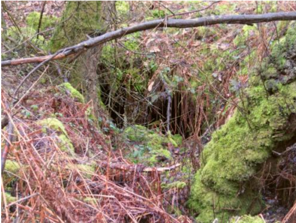
Probable collapse into Vallets Level (SO 6010 1138) looking west
